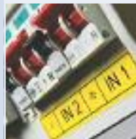
Distribution boxes & patch panels
