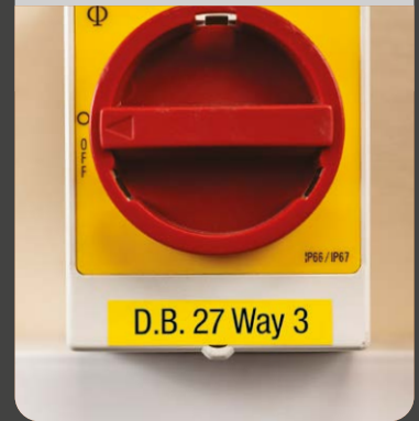
Control gear and switchgear
