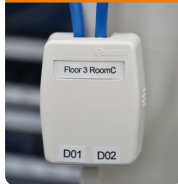
Equipment and telecoms outlet
