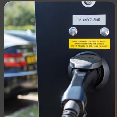
EV charging / Solar
